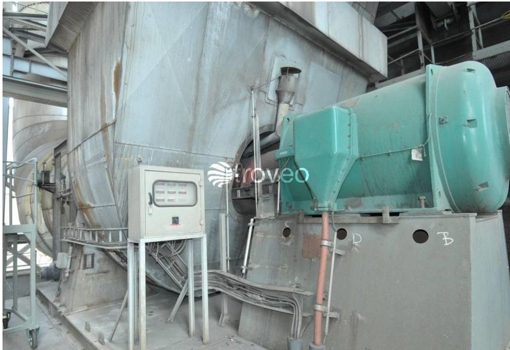
flue gas draft fan system
