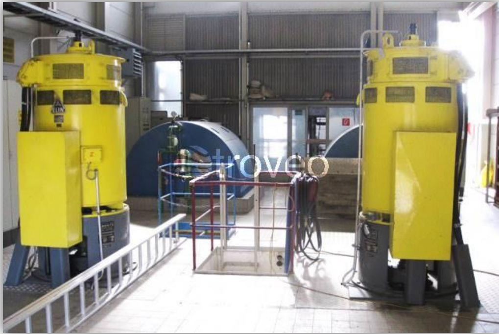
cooling water supply system (water derived from river)
