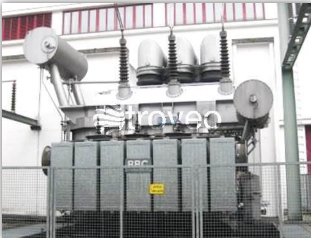
main step-up transformer
