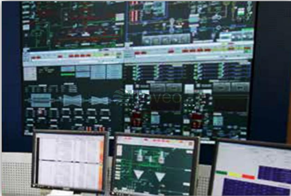
modernised control centre
