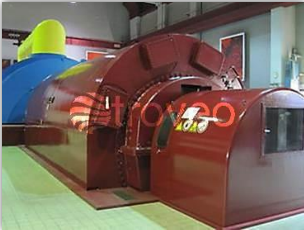
steam turbine – power generator set
