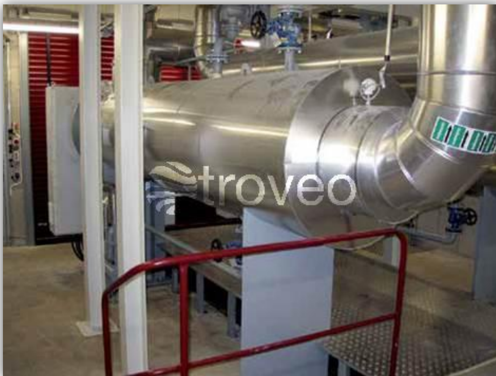
electric heat exchanger
